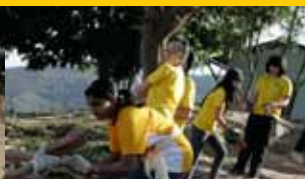
All students and teachers forming a long human chain to transport sand and bricks from hill bottom to hilltop for building of new classrooms.
